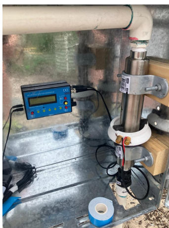
PW75 unit with FG-200 scalar generator (432.00 Hz)
